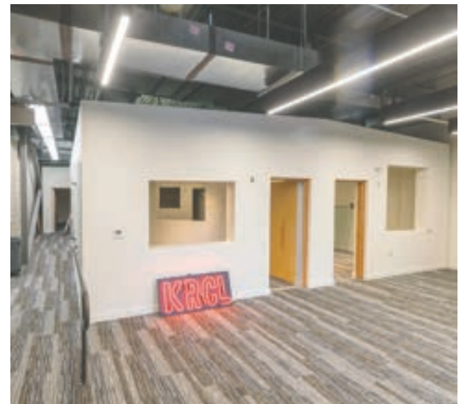
PHOTO COURTESY OF SAM CRUMP PHOTOGRAPHY KRCL’s future On-Air Studios, band room and production studios at 535 West 300 North.
